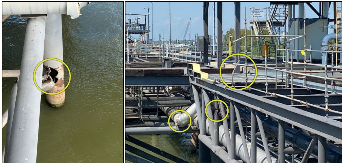
Figure 5. Left to right: Damage to a vertical piling and insulated pipe, pier support bracings, and railing (indicated by the circles). (Source: Coast Guard)
